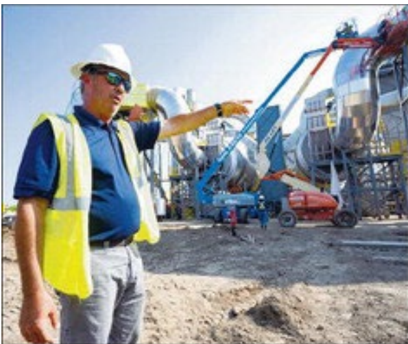
Plant manager Jason Nugent talks about the construction of the Delta Biofuel facility in Jeanerette on Aug. 12.
