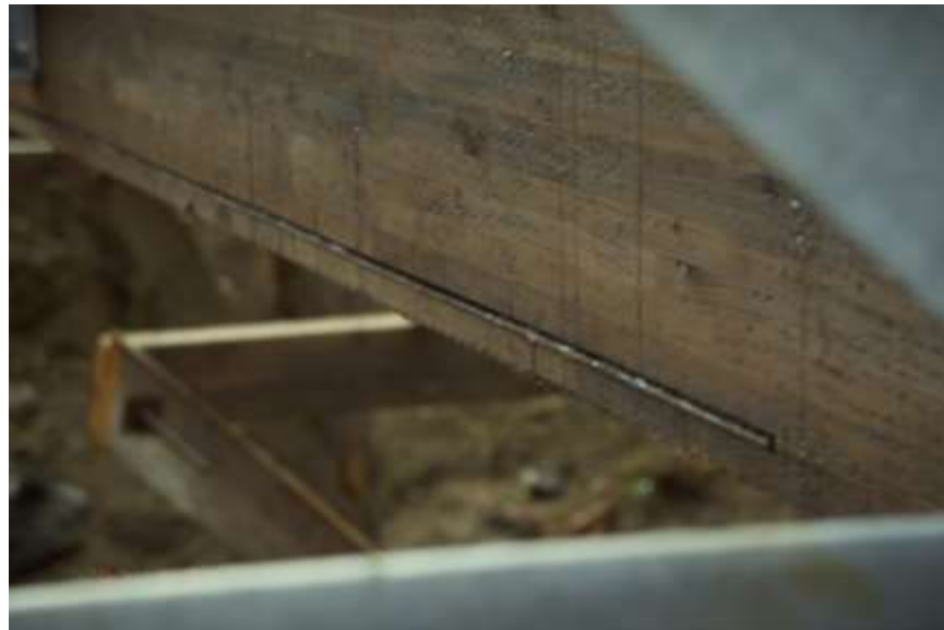
Figure 4-28: The glulam girders are reinforced with a layer of fiber-reinforced polymer (FiRP®) which permitted a significant reduction in the volume of wood required compared to an unreinforced bridge. This bridge has been in service since the early 1990's.
