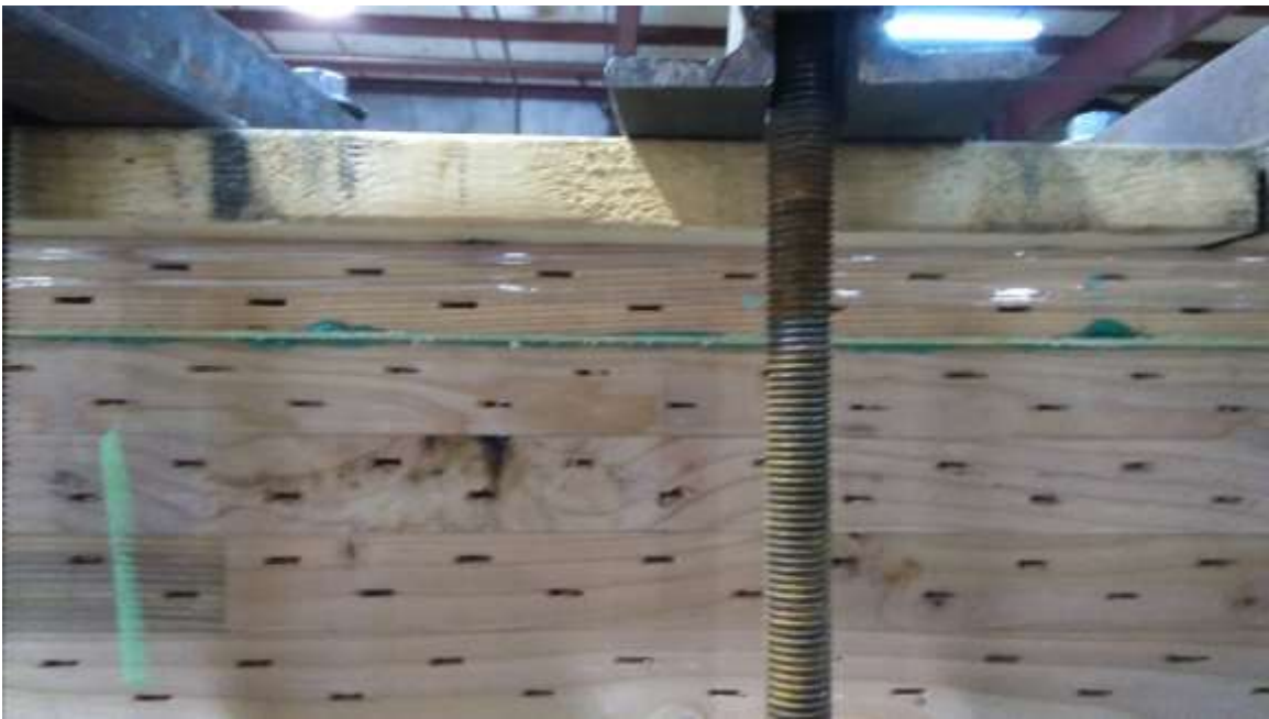
Figure 4-16: The glulam girders are reinforced with high-strength fiber on the tension face. This fiber-reinforcing is installed in the shop prior to assembling the structure.
