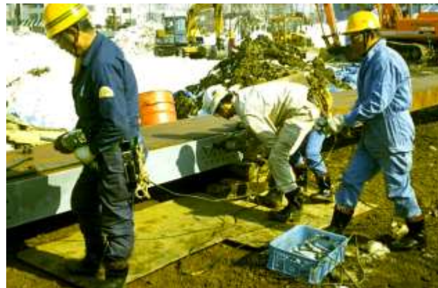
Figure 4-42: The new glulam superstructure was preassembled using 12 meter long sections of high strength fiber reinforced glulam beams. The bridge had a 1 meter depth girder limitation and high strength fiber reinforced glulam beams were the only economical option. This structure has been in place close to twenty-five years.
