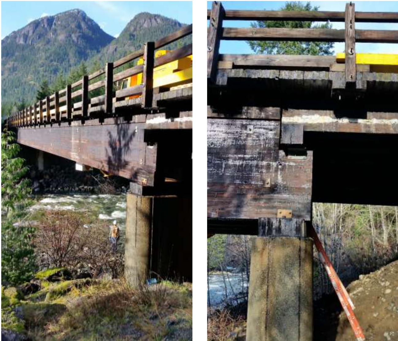
Figure 4-8: Elk River Bridge consists of six glulam I-beams spanning 35m; at each end is an approach span of approximately 8m made up of solid sawn girders. The deck is transverse nail-laminated timber.
