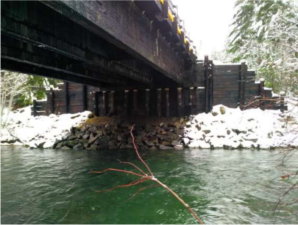
Figure 4-9: Cervus Creek Bridge is a 25m (82ft) single-span bridge consisting of four glulam I-beams with a transverse nail-laminated deck.
