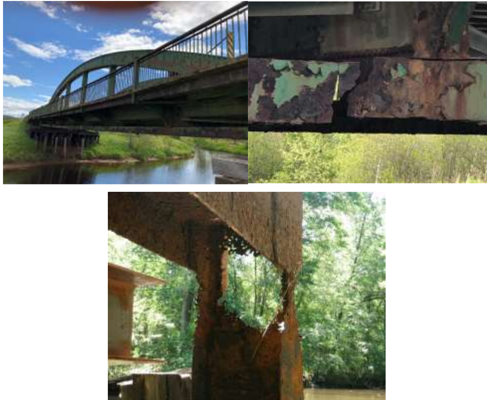
Figure 4-14: Photograph of the existing steel arch span that will be replaced by the new timber structure shown in Figure 4-13. Middle photograph shows the rusted through tension cords (out of service) in the old bridge that was less than 50 years old. Steel has not yet solved its rust problems with rust resistant steel particularly in marine environments where a patina of moisture that stays in place over prolonged periods. In such cases rusting of less than 25 year old elements like the bottom photo reveals have been found to occur. Bottom photograph of rust resistant steel in a railway bridge in Georgia near the coast. Wood doesn't rust!
