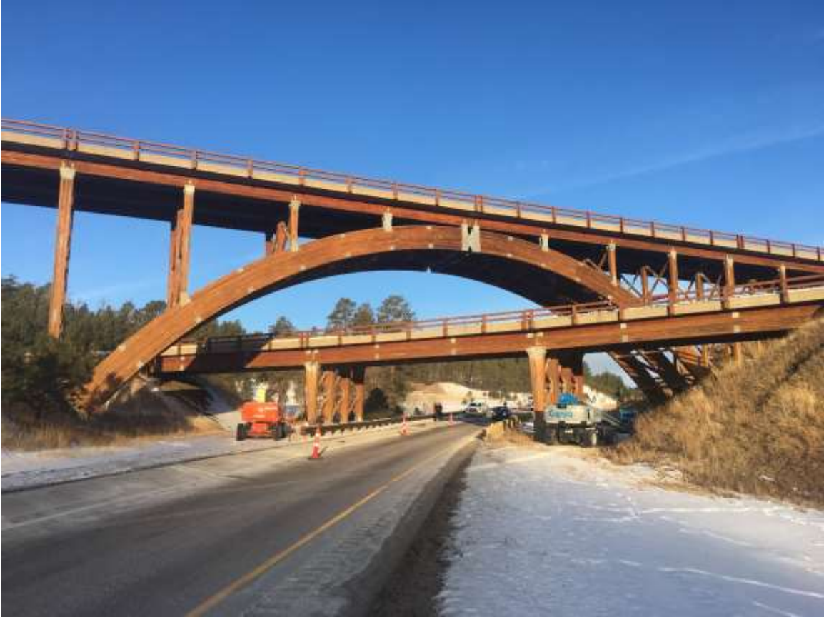
Figure 4-1: The Keystone Wye Bridges in South Dakota were recently inspected after more than 50 years in service, and were found to be in good condition; only minor repairs and routine maintenance were recommended to extend the longevity of the structures.
