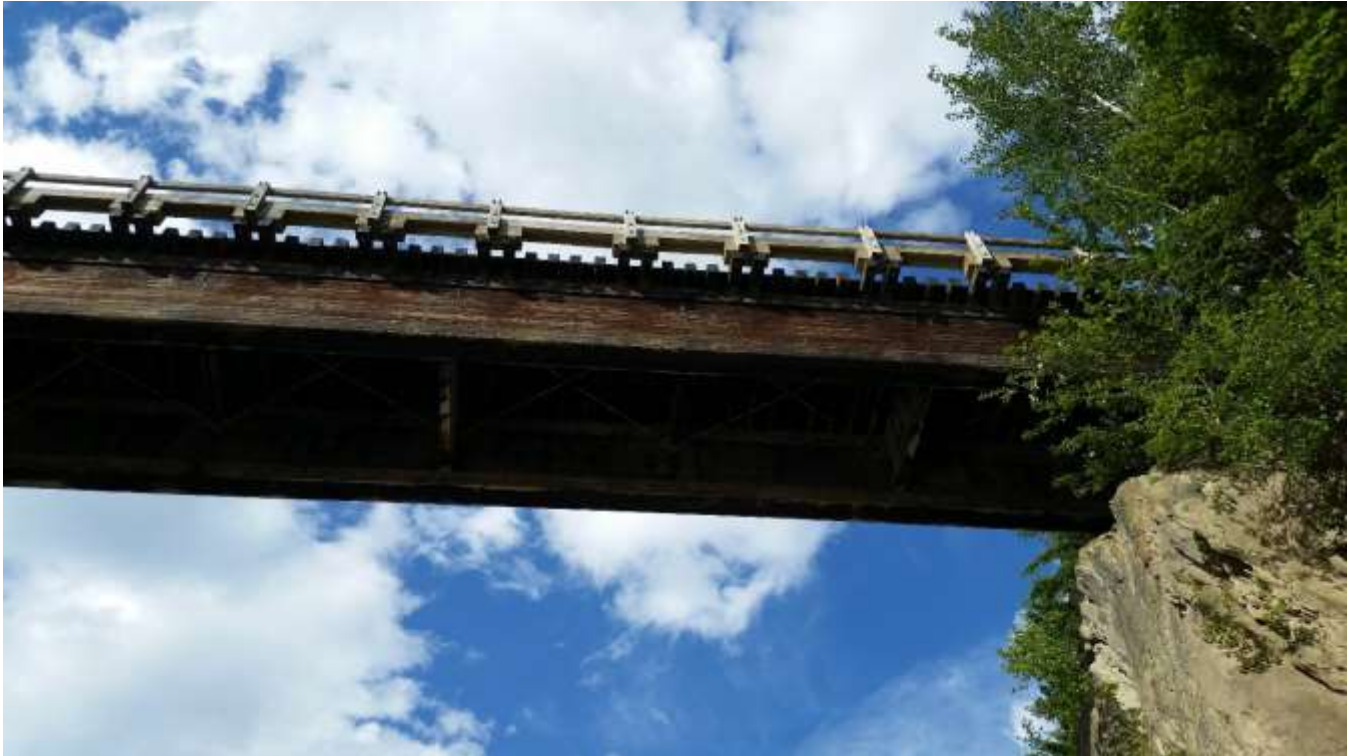
Figure 4-7: A recent inspection of the bridge found it to be in fair condition overall. The only significant deficiencies found were in the deck system as a result of vertical fasteners allowing water to penetrate into the timber elements. Even with these deficiencies, the bridge can maintain an L100 load rating. Recommendations were given for repairs and maintenance that could extend the life of the bridge for as much as 80 more years.
