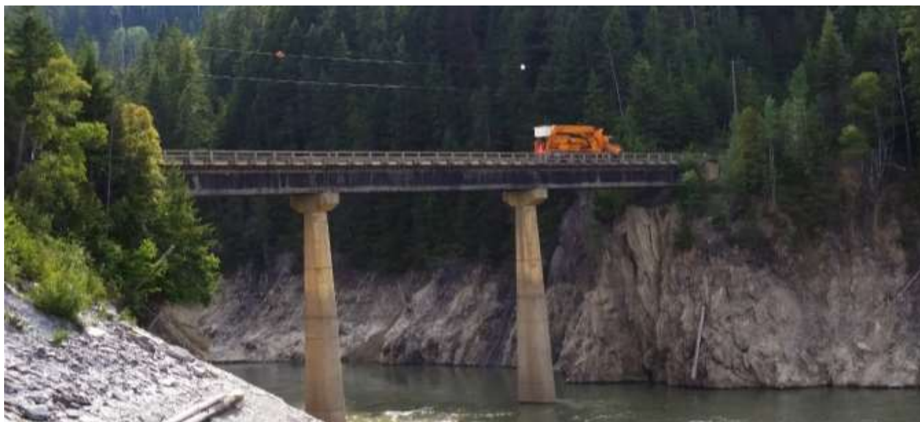
Figure 4-5: Golden Bridge, in British Columbia is a 3-span glulam timber bridge, totaling 82m (270 ft) in length.
