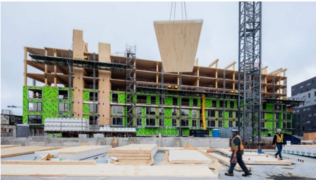
Construction using CLT at the Arbora Complex in Montreal, Quebec. Source: Nordic Structures
