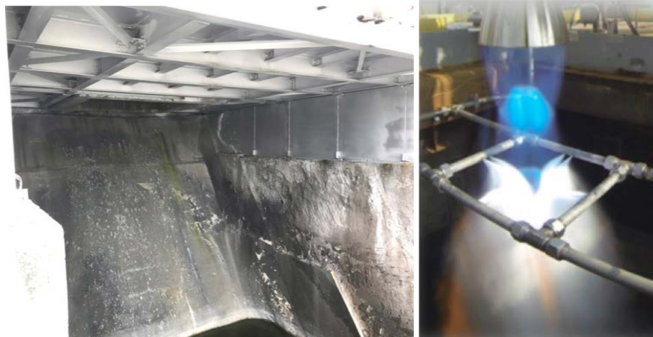
Figure 4: Left: Damage caused to uncooled flame trench, NASA SSC. April 26, 2017, Right: Water spray ring used to cool Morpheus engine static test [7].
