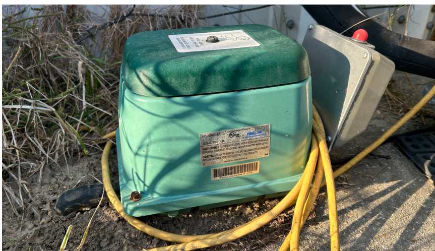
Residential septic aerator in area of potential flooding. Photo by Richard Grabert
