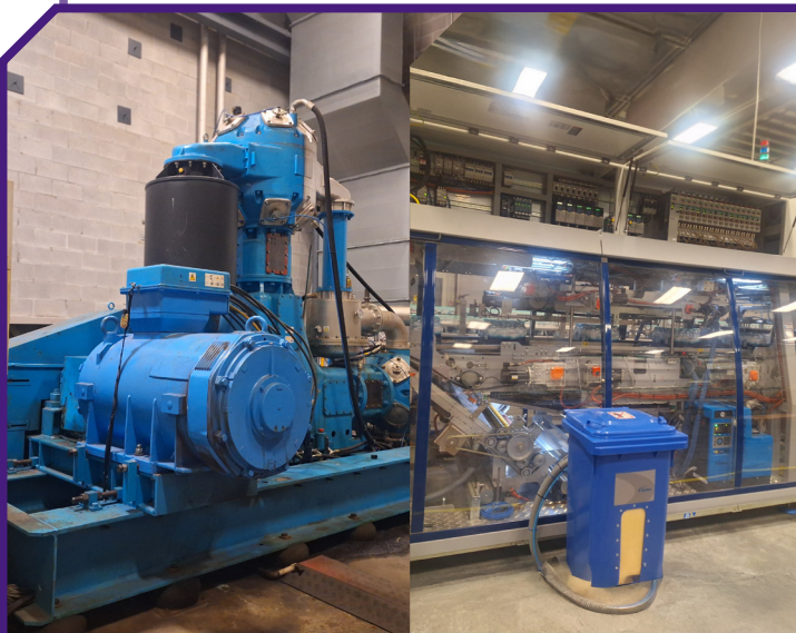
Large pumping systems offer water and energy savings opportunities. Photo by LSU ITAC students
