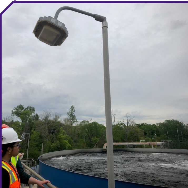
Outside lighting around clarification tanks can be switched for energy savings. Photo by LSU ITAC students
