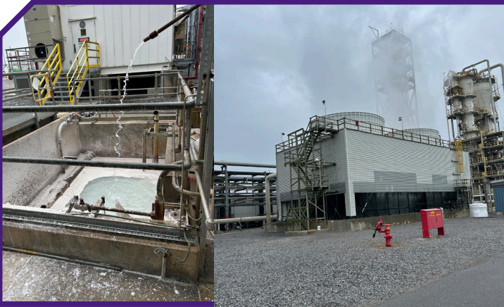
Water collection and cooling towers have opportunities for sustainability
